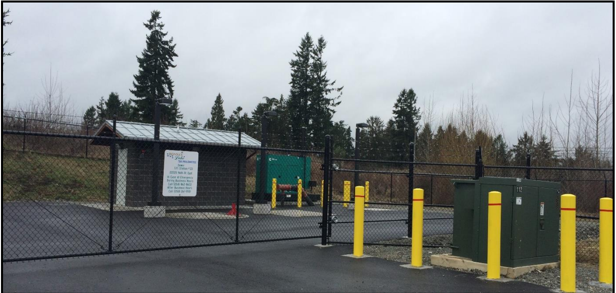
Lift Station No. 23
